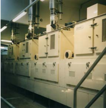
Photo: 4 x 25kW units used for Drying of Bread Loaves before Slicing
